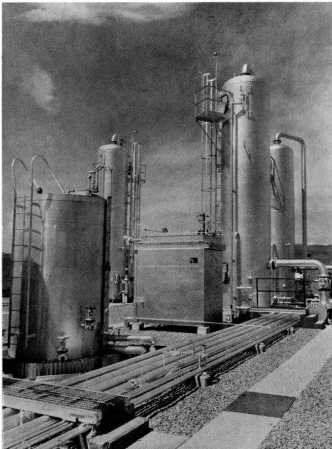
ABOVE GROUND FACILITIES at PSCo's Leyden Mine Gas Storage Project. This was the first abandoned coal mine known to be used for underground storage of gas.
