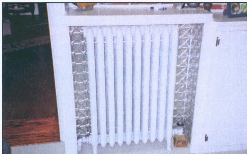
Figure 25. Hot Water Radiator in Restored Home on Warm Springs Avenue (photo by author, 2006)
