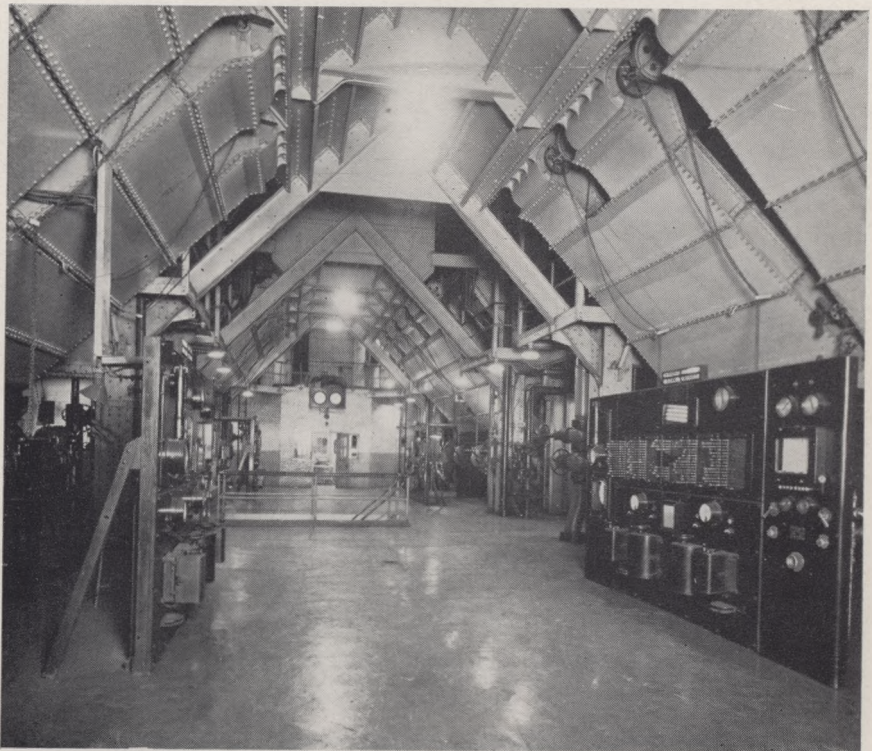
Fig. 11—Boiler Room, Beacon Street Heating Plant
